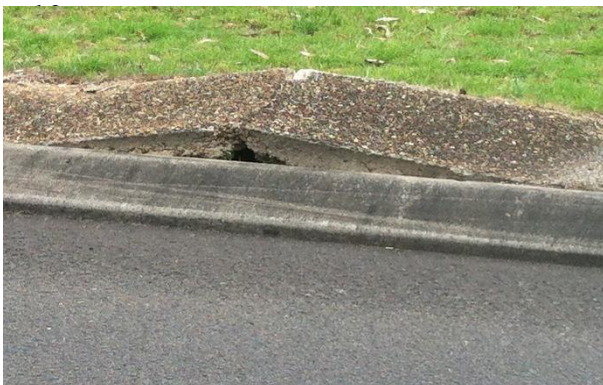
Figure 1. Pavement upheaval (source: author)
