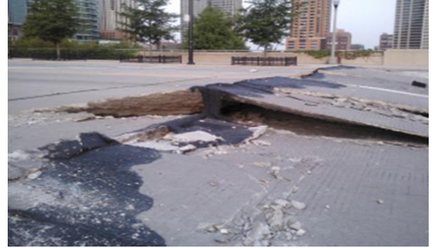
Figure 4. Buckled pavement (CBS Chicago 2012)
