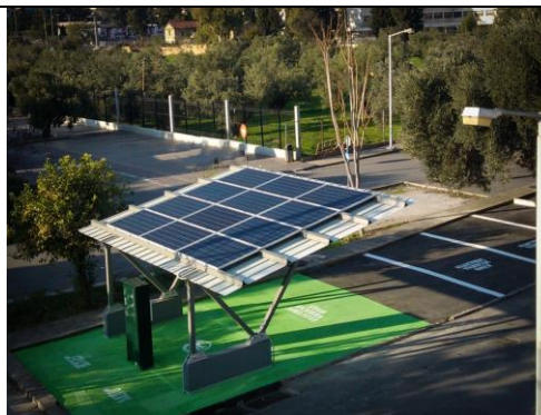
Figure 2. UNIWA solar EV charging station.
